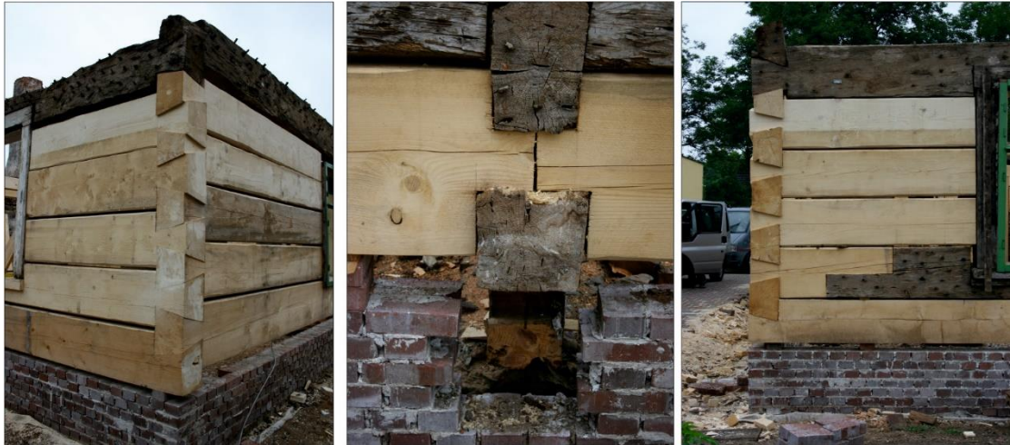
Fig. 4: Rehabilitation of elements and joints of timbered wall using the classic method – replacement, sealing
