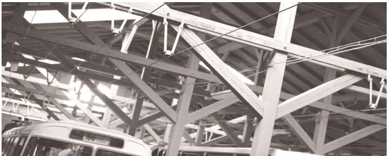
Fig. 3. Wooden skeleton in Public Transport Museum located in the tram depot Prague-Střešovice (author's photo)
